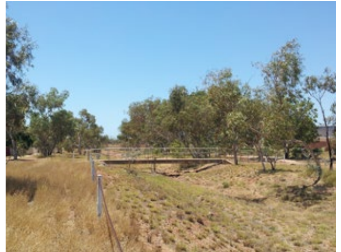
Image 74. Existing drainage swale in Millars Well
