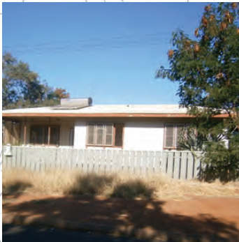
30+ Years Poor Condition
